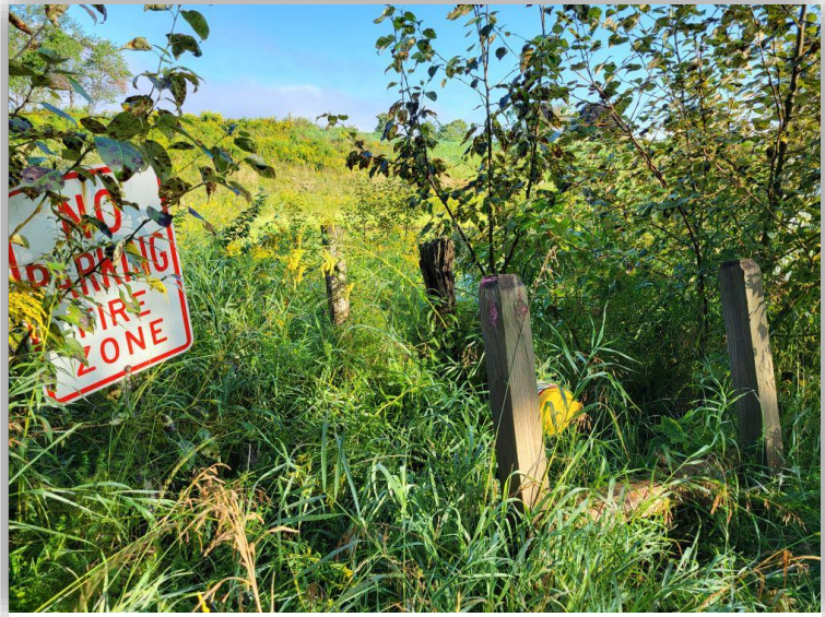
Gore Road Dry Hydrant, Photo Credit - Stacy Boone
